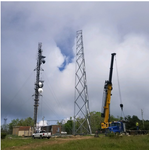
New Bucks Elbow Mountain tower construction in progress next to the existing tower.
