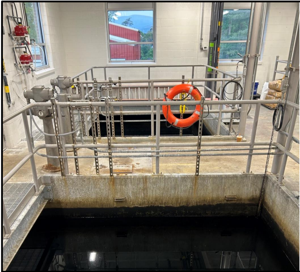
Filters at Crozet Water Treatment Plant
