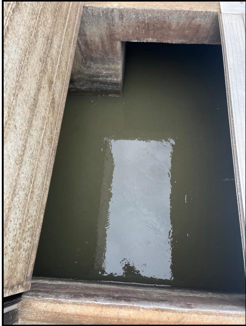
Sewage entering wastewater plant
