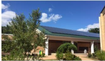
Rooftop solar installation at Mary Carr Greer Elementary School in Albemarle County.
