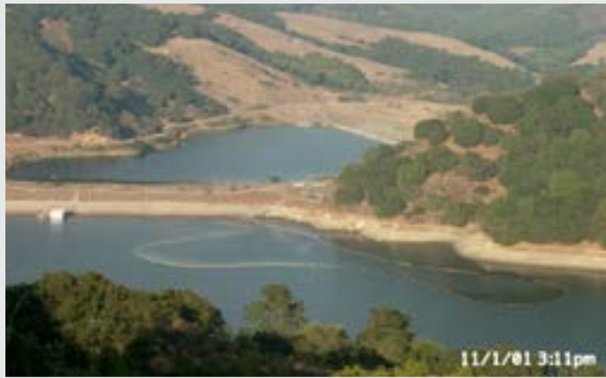
Mobley system installation in Upper San Leandro Reservoir, CA
