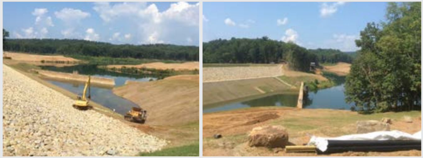
Left: View of old Ragged Mountain Dam from left abutment of new dam August 5, 2014 Right: New Ragged Mountain Dam and old dam to the right August 5, 2014
